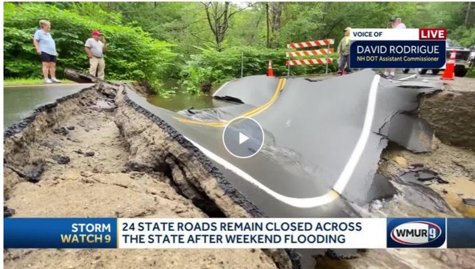
Figure 1-1 Result of a Failed Culvert in Alton 1
